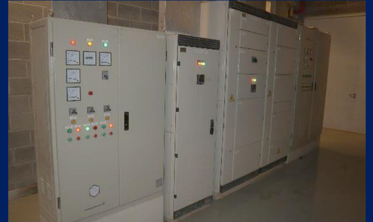
Panel Chiller Room
