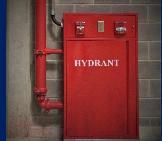
Indoor Hydrant Box
