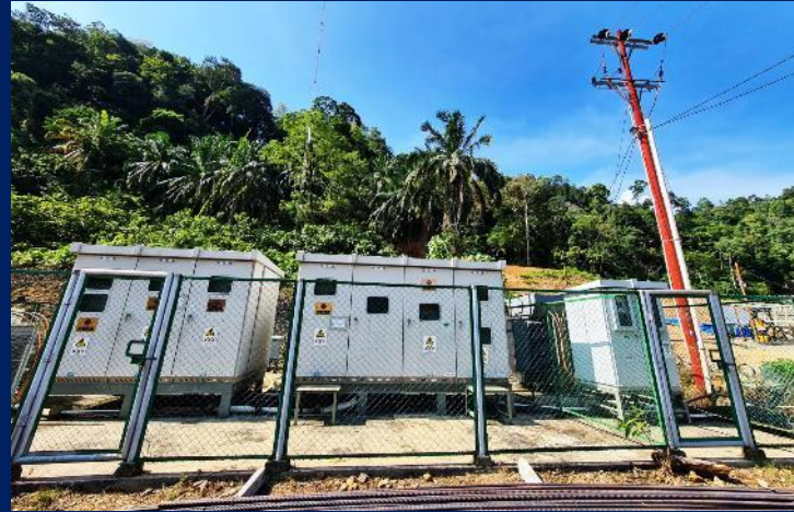
Distribution Line Pole 20kV
