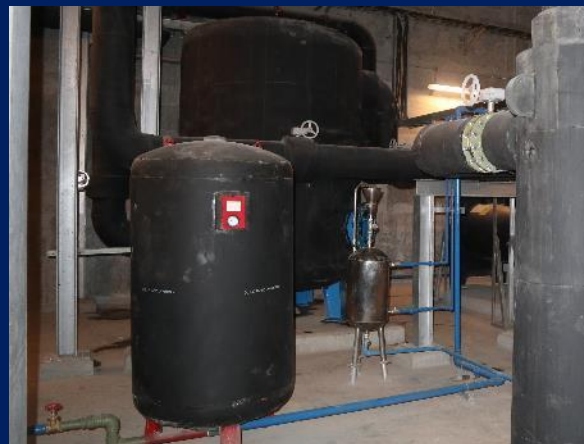
Buffer Tank & Expansion Tank
