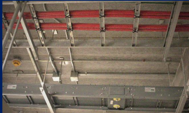
Feeder Cable To Transformer
