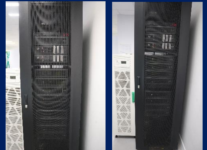
Cabinet Rack Sound System
