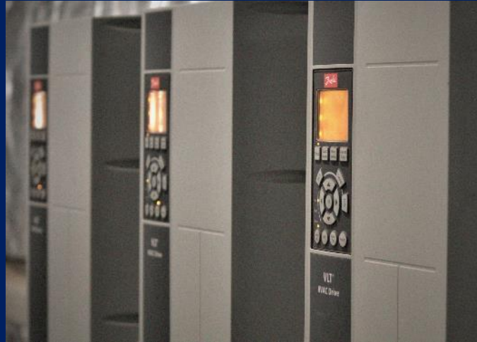
VSD Cooling Tower
