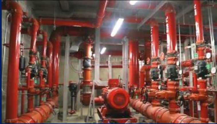
Fire Hydrant Pump
