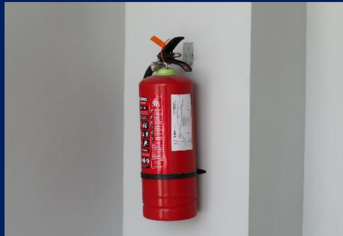
APAR / Fire Extinguisher
