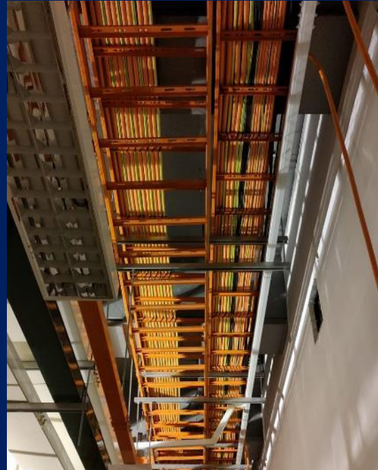
Feeder Cable MV
