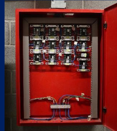
Terminal Block Fire Alarm
