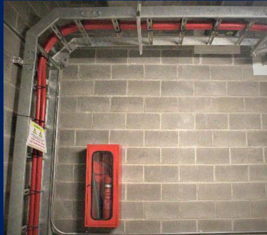
Feeder Cable To MVMDV
