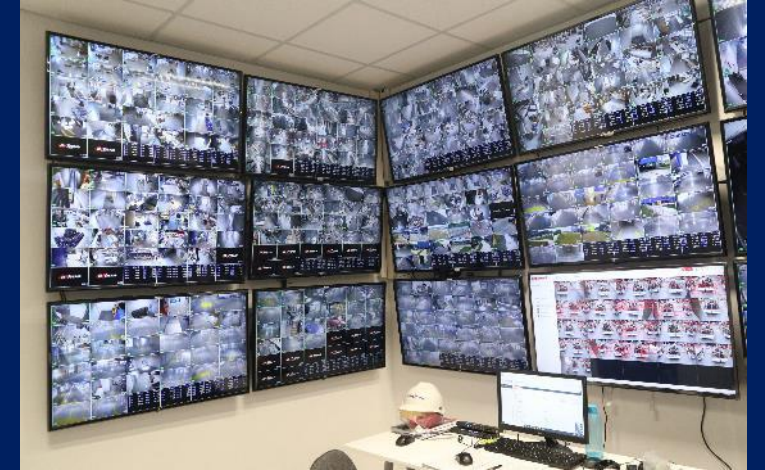
Control Monitoring CCTV
