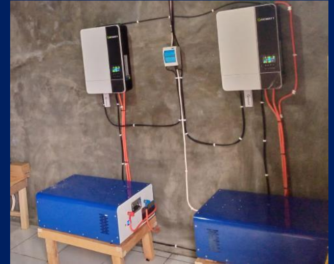
Inverter & Battery System
