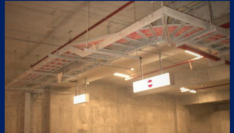
Feeder Cable MV
