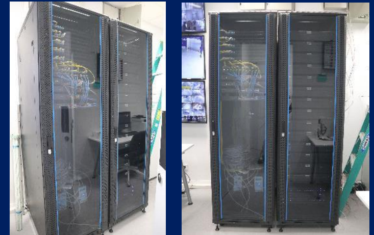
Cabin Rack NVR
