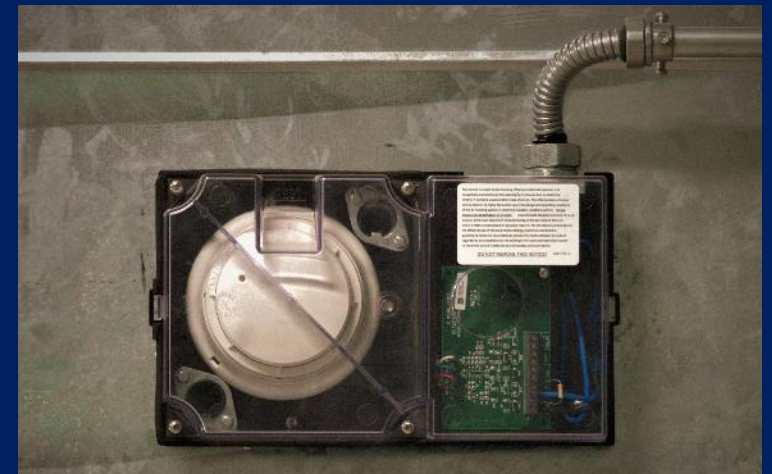
Duct MH Sensor
