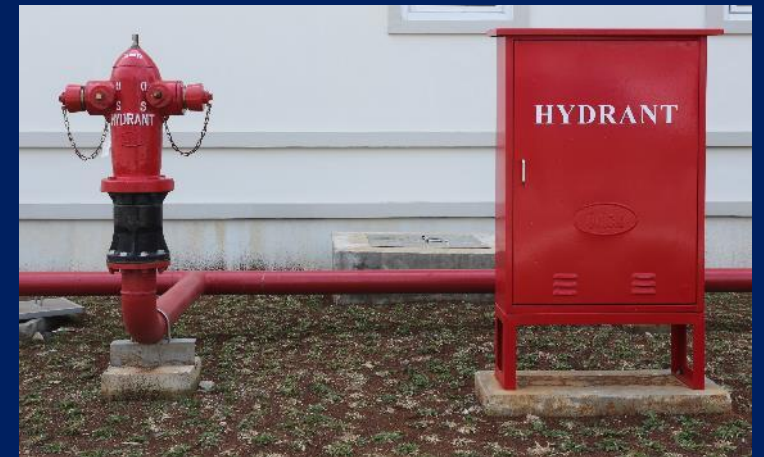
Hydrant Pillar & OHB
